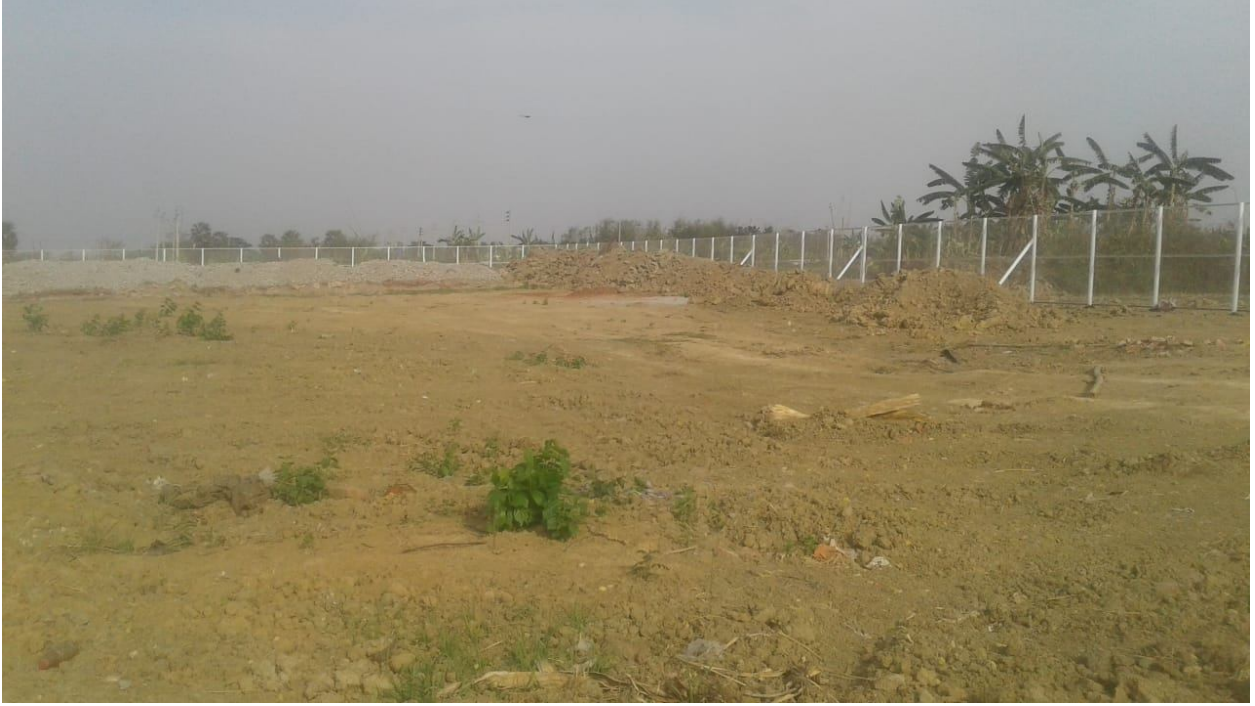
01 Apr 2020 : Boundary Fencing
