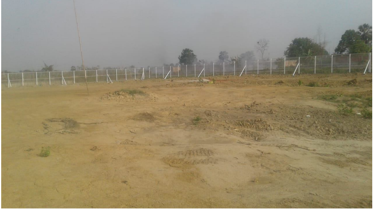
01 Apr 2020 : Boundary Fencing
